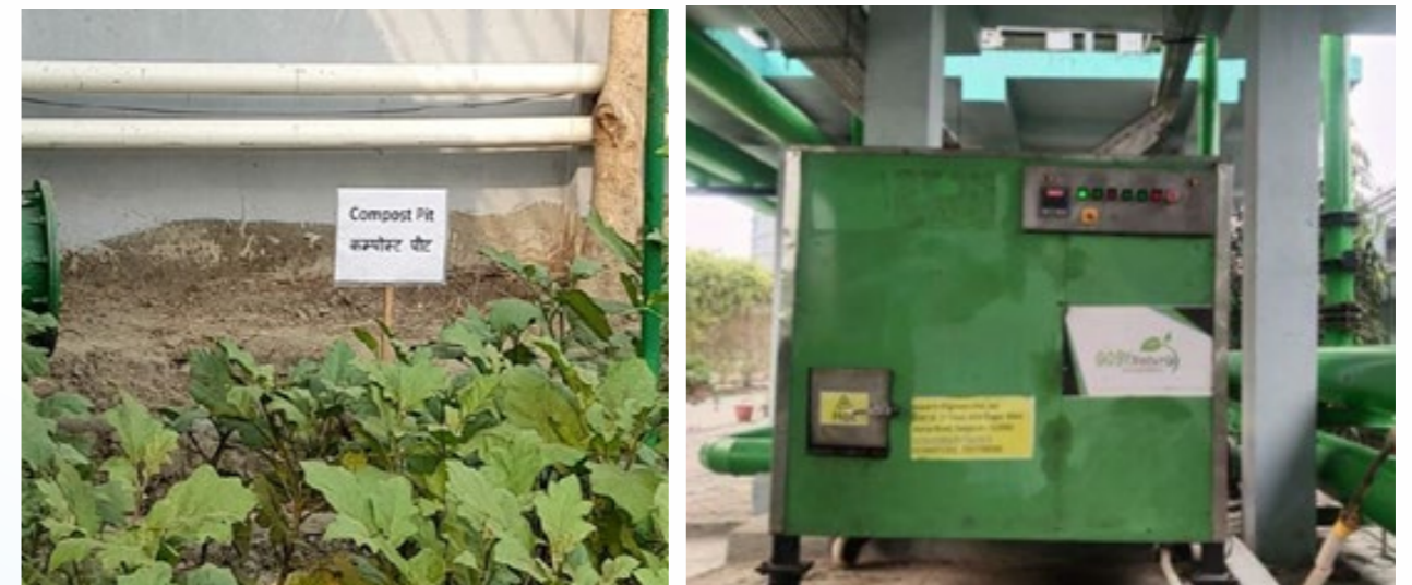
Compost pit and machine installed for the recycling of waste at SBIL, Kolkata
